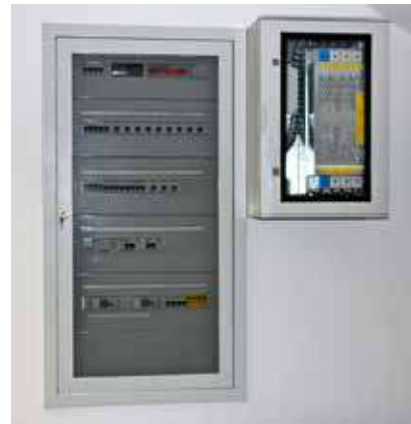
Data Center Protection realised with an ILF 4P 250, installed in the course of refurbishment.
