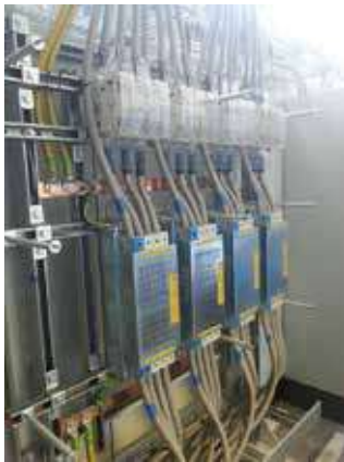
Data Center Protection realised with 4 parallel connected ILF 4P 400 SPDs.
